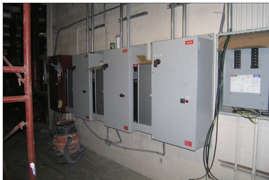
Architectural & Engineering Services- Electrical Panels
